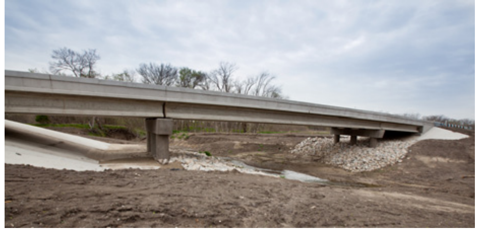
Looking south along Slayter Creek at the new Outer Loop frontage road bridge. The trail “bench” is visible under the bridge on the left side of the image.
