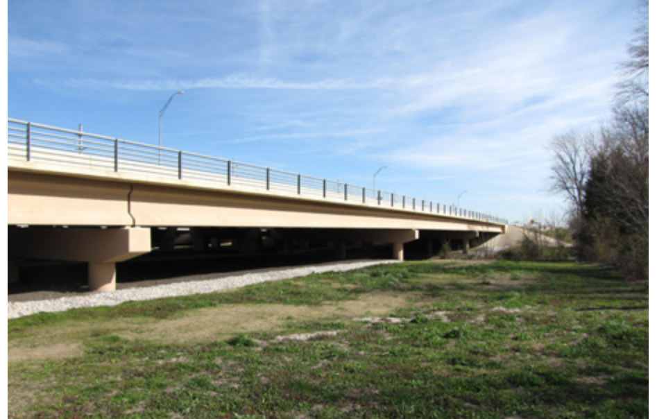
Looking northeast at the State Highway 121 bridge. The creek crosses under the bridge on the far side of the row of columns near the middle of the image.
