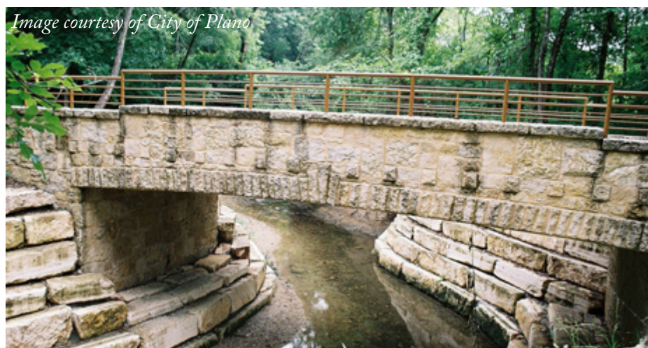
The maintenance of creek crossings is an important consideration, as heavy rain can cause significant levels of sedimentation and debris build-up.
