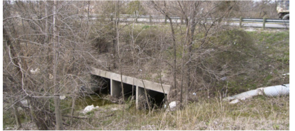
Roadways crossing creeks can be both opportunities and constraints for trail connections. In this instance, the use of culverts rather than a bridge structure precludes the possibility of a trail crossing under the roadway along the creek.
