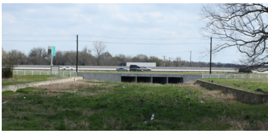
This is an example of a missed opportunity for a trail crossing under SH-121.
