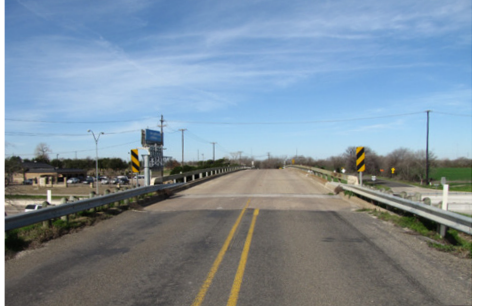
Looking west at the existing Ridgeview Drive bridge over US-75. The current bridge is too narrow for a trail connection.
