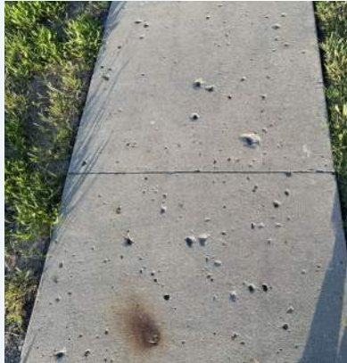
Walking paths show signs of deterioration and concrete pitting.
